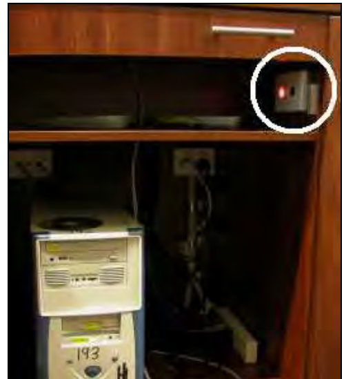
Master power switch
